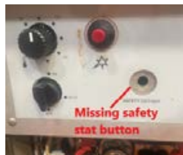
Gas fryer – safety stat reset button damaged/missing.
